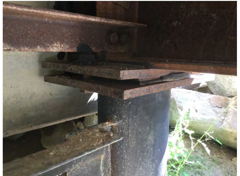
Rubber bearing slight bulge
