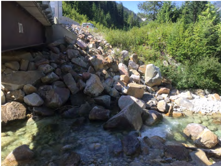
Down stream left bank rip rap scour
